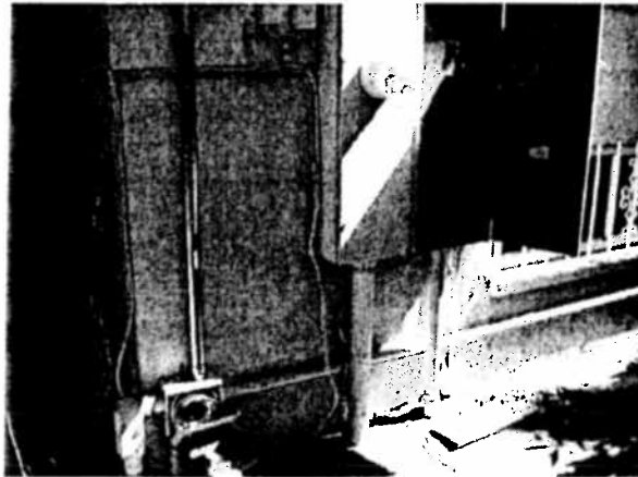
Electrical service alongside the south side
